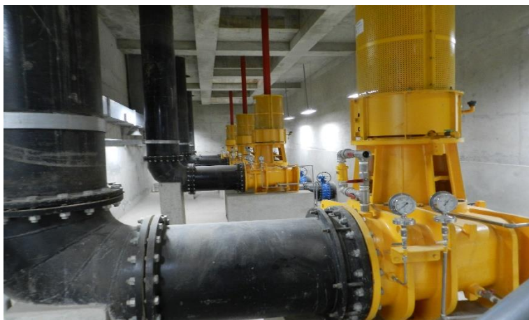
Completed Installation of Transmission Pumps including Valves, Pipes and Fittings at Pump Station
